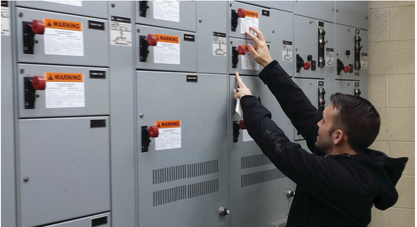
Labeling equipment at Lower Creek WWTP, City of Lenoir
