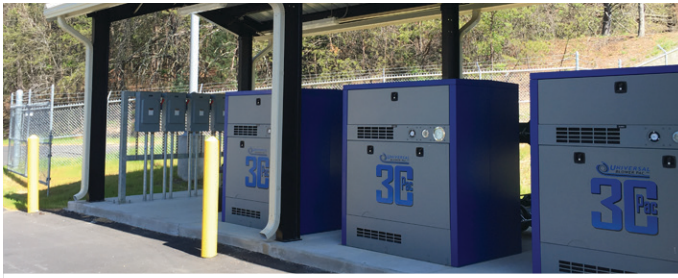
Blowers at Gunpowder Creek WWTP
