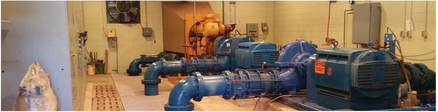
High service pump station at Valdese WTP.
