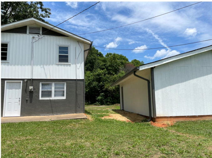
Above: View of 2110-A Walt Arney Rd (Lot 2) from rear yard. Note locations of the concrete patio and the interior door to the outbuilding.
