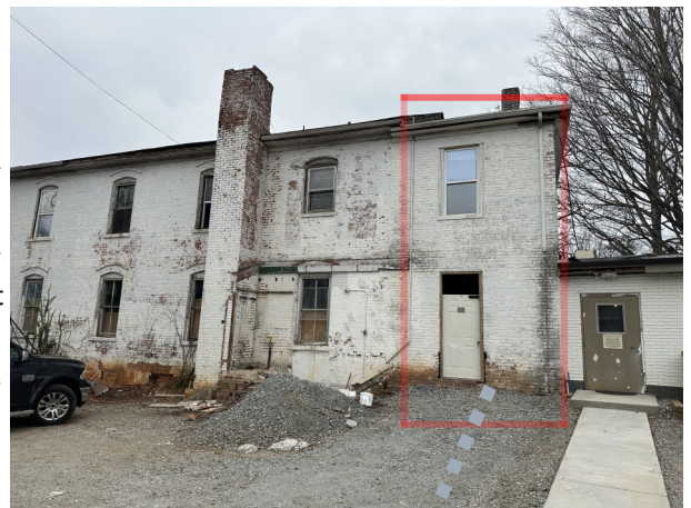
Above shows 10' wide area to be demolished to allow for building separation and new rear lot line.
