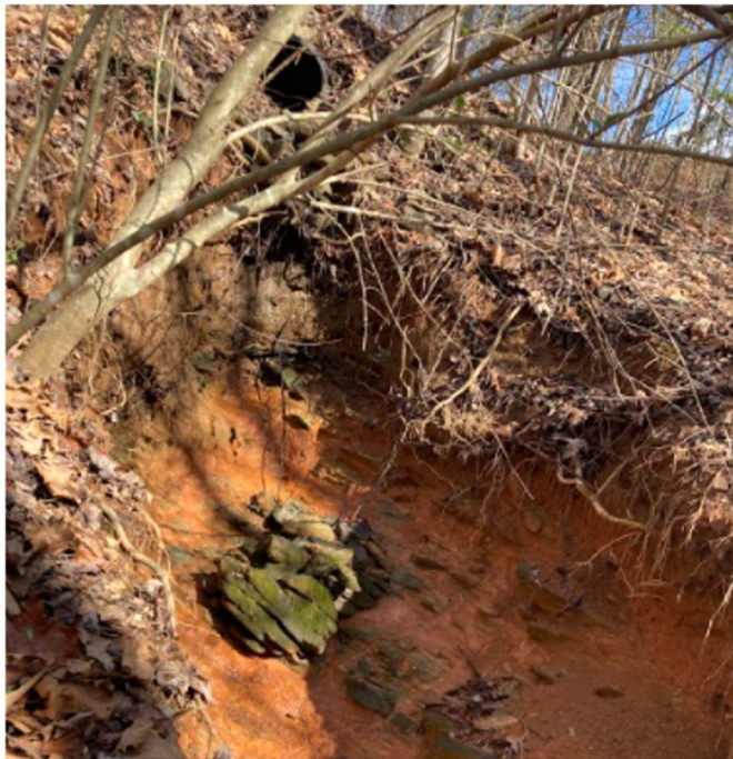
Erosion on Lot 29 below the outfall
