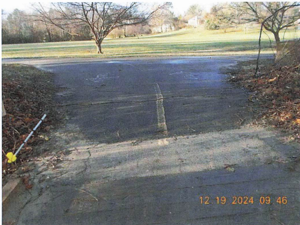
UP TO 6" OF SETTLEMENT IN WEST APPROACH
