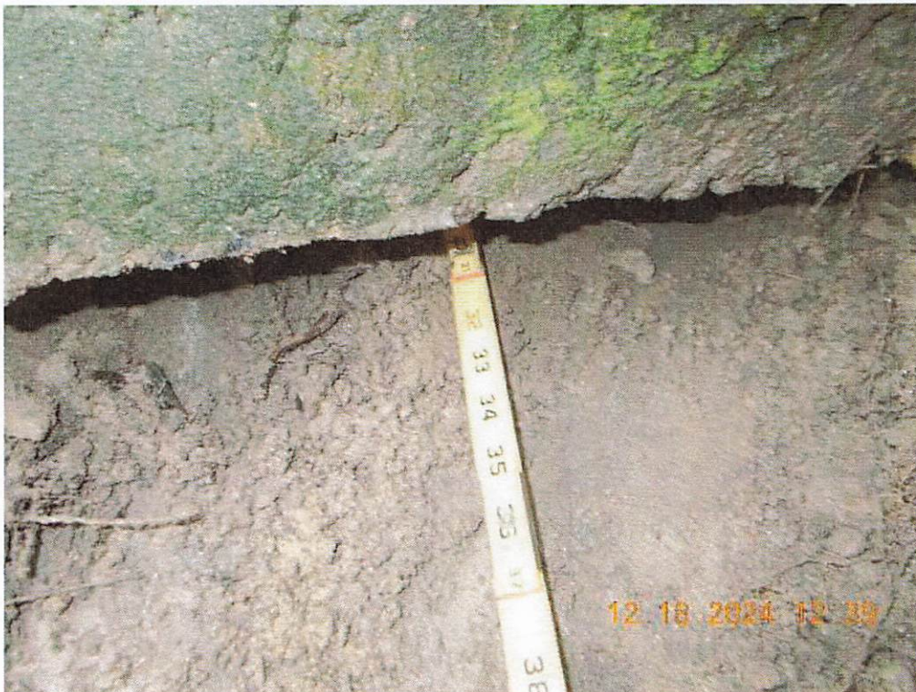
EROSION/ SCOUR, ABUTMENT 1 FOOTER, 4" HIGH X 2'-8" DEEP ✓
