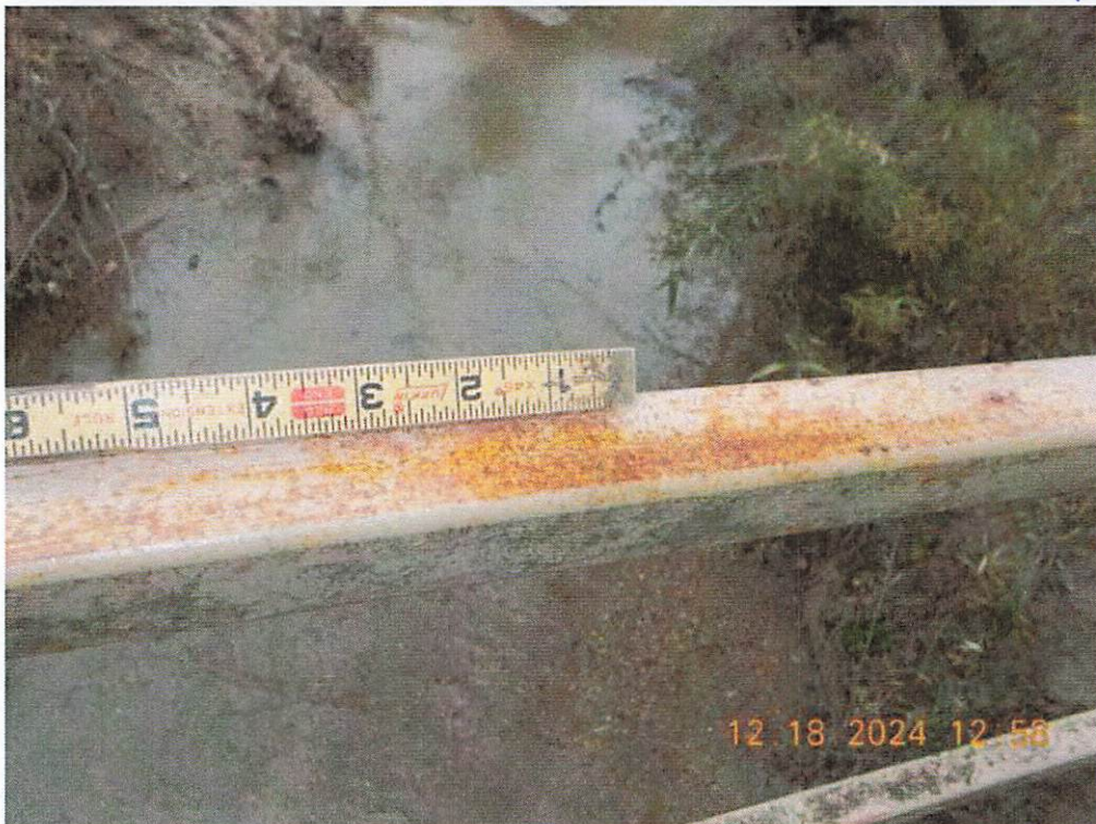
SCATTERED SURFACE RUST TO RAILS
