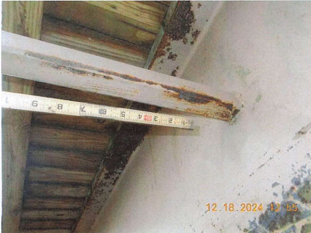
SCATTERED PAINT PEELING WITH SURFACE RUST TO POST BLOCK SUPPORTS
