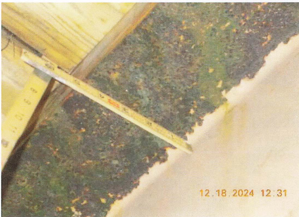
PAINT PEELING, SURFACE RUST, TOP FLANGE ⇐ Not by the event.
