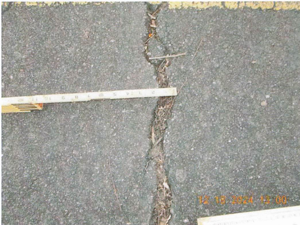
2" WIDE CRACKING IN WEST APPROACH, ABUTMENT 1
