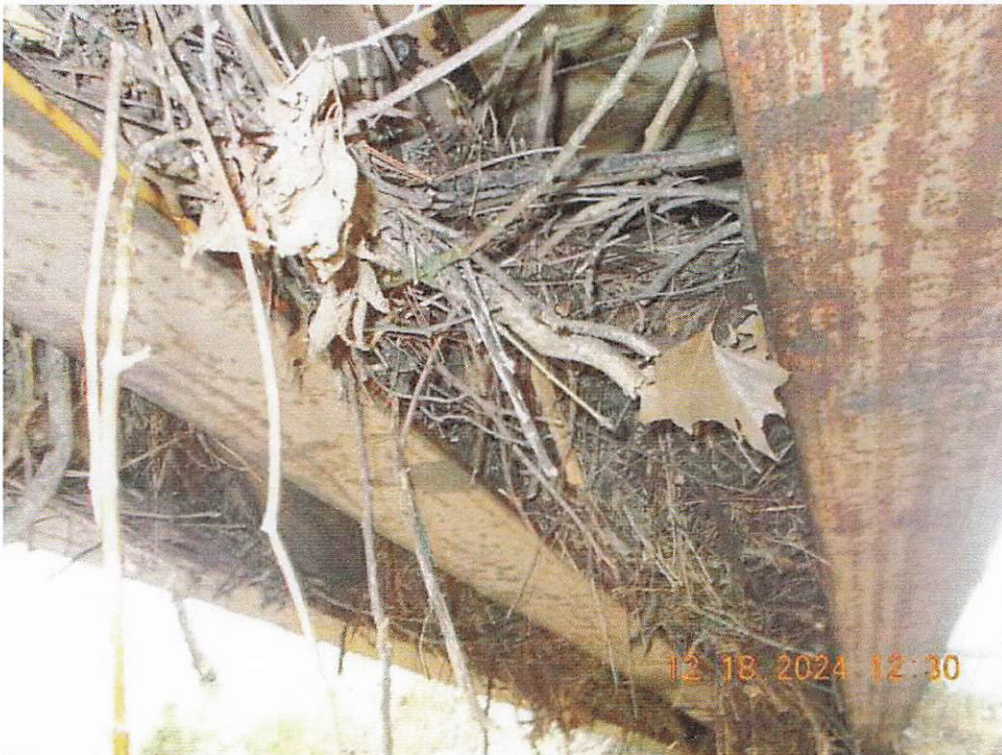
DEBRIS BETWEEN BEAMS ✓
