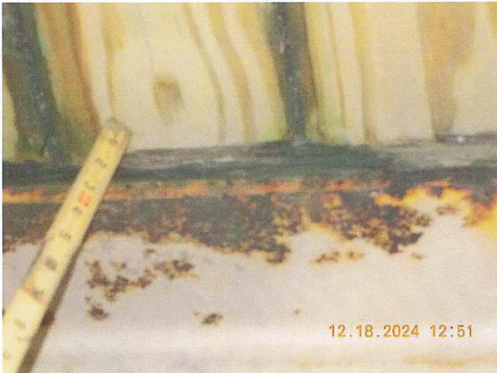
DECAY IN NAILER 1, 1'-8" LONG X 2" HIGH X 1" DEEP, 10'-0" FROM ABUTMENT 2
