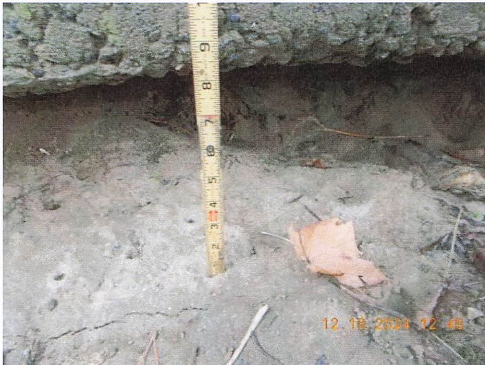
VOID/ SEPERATION, 8" HIGH X 2'-0" DEEP X 10'-2" LONG X 2'-8" UP FROM GROUND LINE ✓
