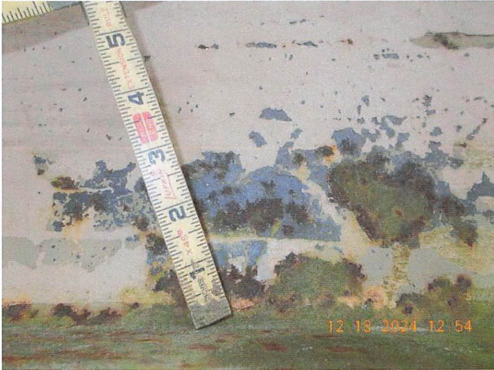
SCATTERED PAINT PEELING WITH SURFACE RUST TO WEB OF ALL BEAMS
