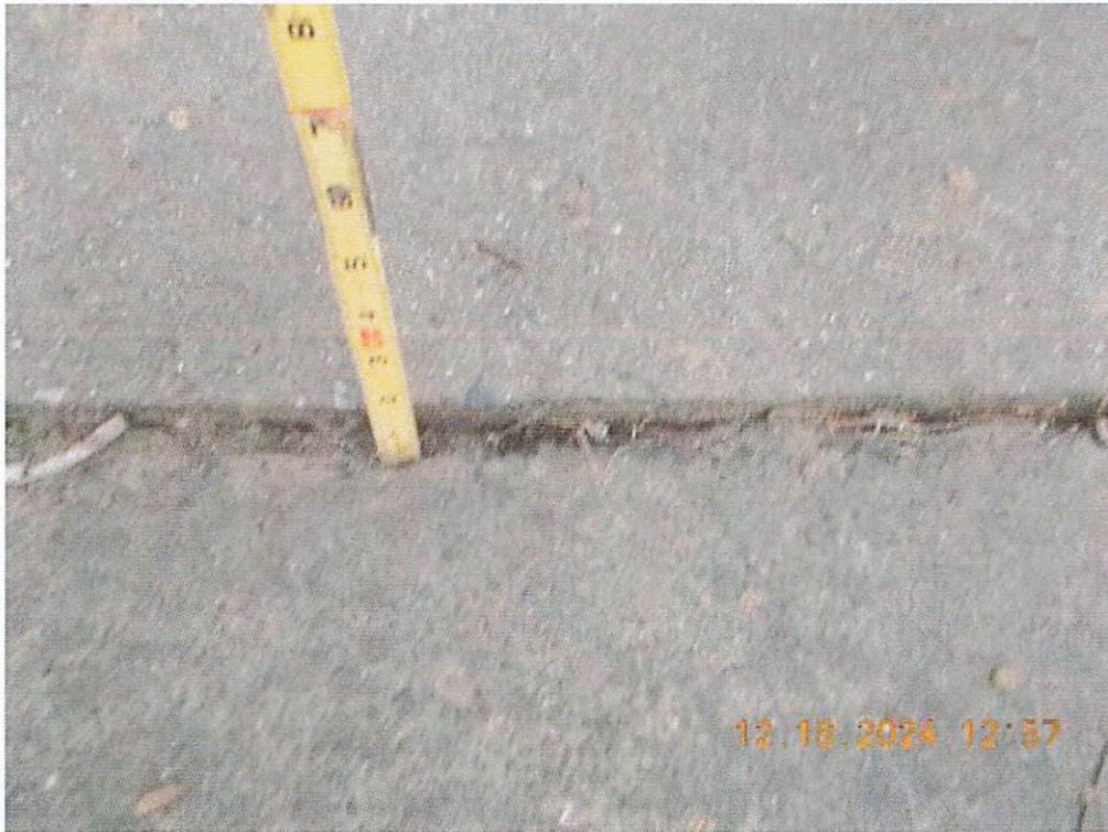
SETTLEMENT IN EAST APPROACH, UP TO 1/2" DEEP
