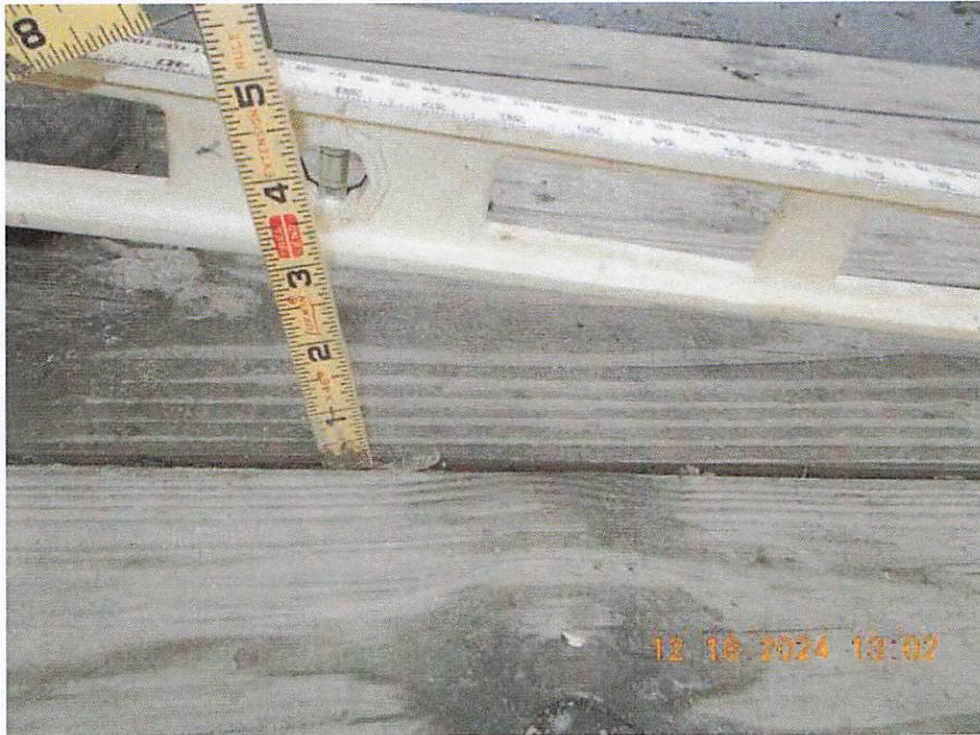
BRIDGE OUT OF GRADE, UP TO 3" AT ABUTMENT 1 ✓
