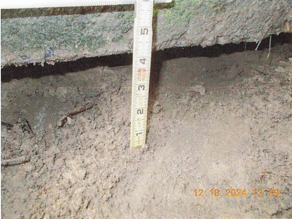
EROSION/ SCOUR, ABUTMENT 1 FOOTER, 4" HIGH X 2'-8" DEEP ✓
