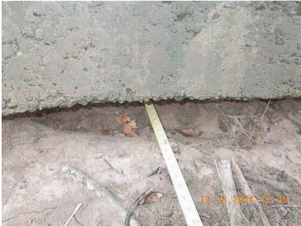
VOID/ SEPERATION, 8" HIGH X 2'-0" DEEP X 10'-2" LONG X 2'-8" UP FROM GROUND LINE ✓
