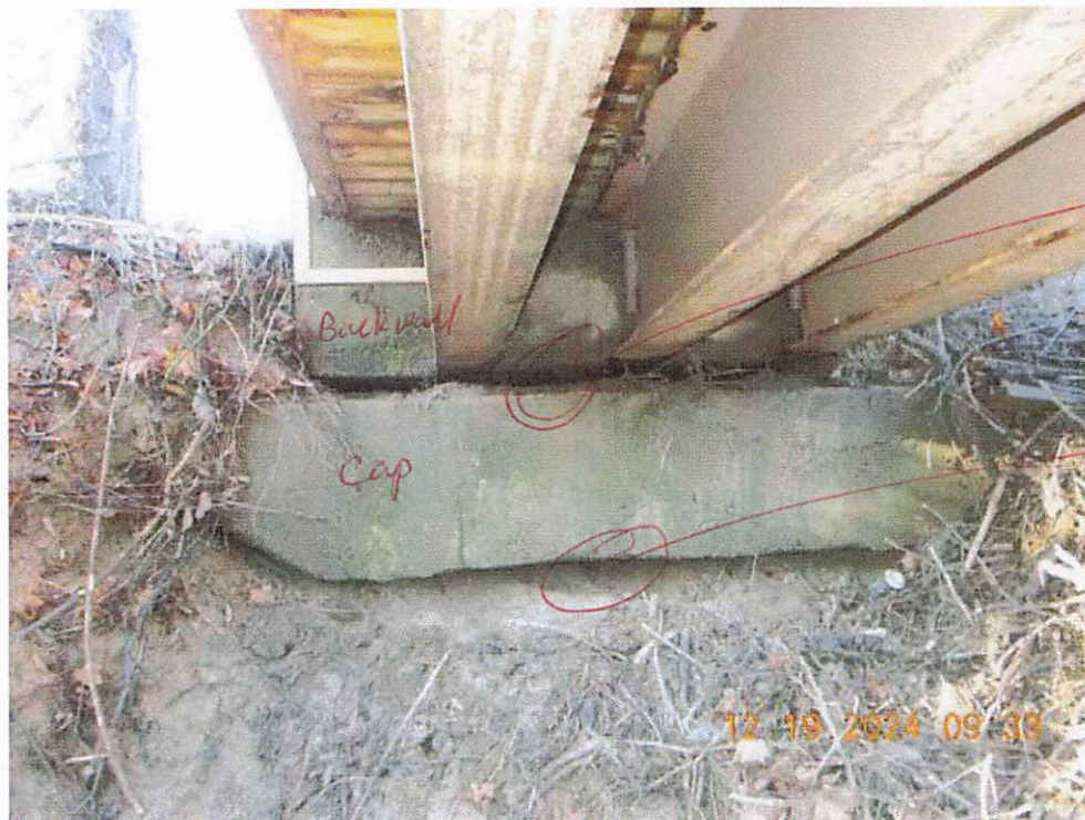
ABUTMENT 1 EROSION/ SCOUR AND 8" HIGH SEPARATION/ VOID BETWEEN CAP AND FOOTER ✓
