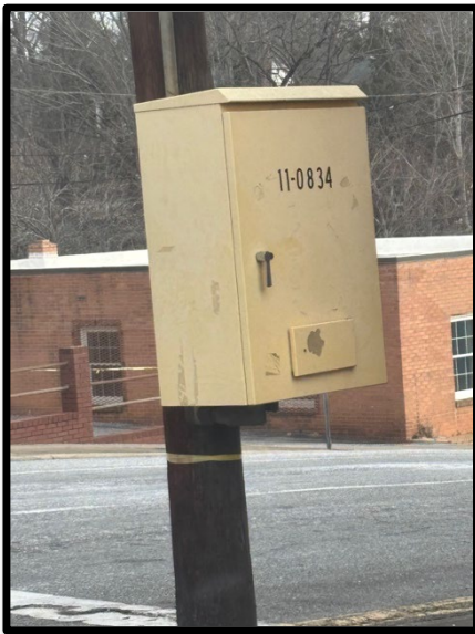
City of Lenoir Traffic Signal Cabinet
