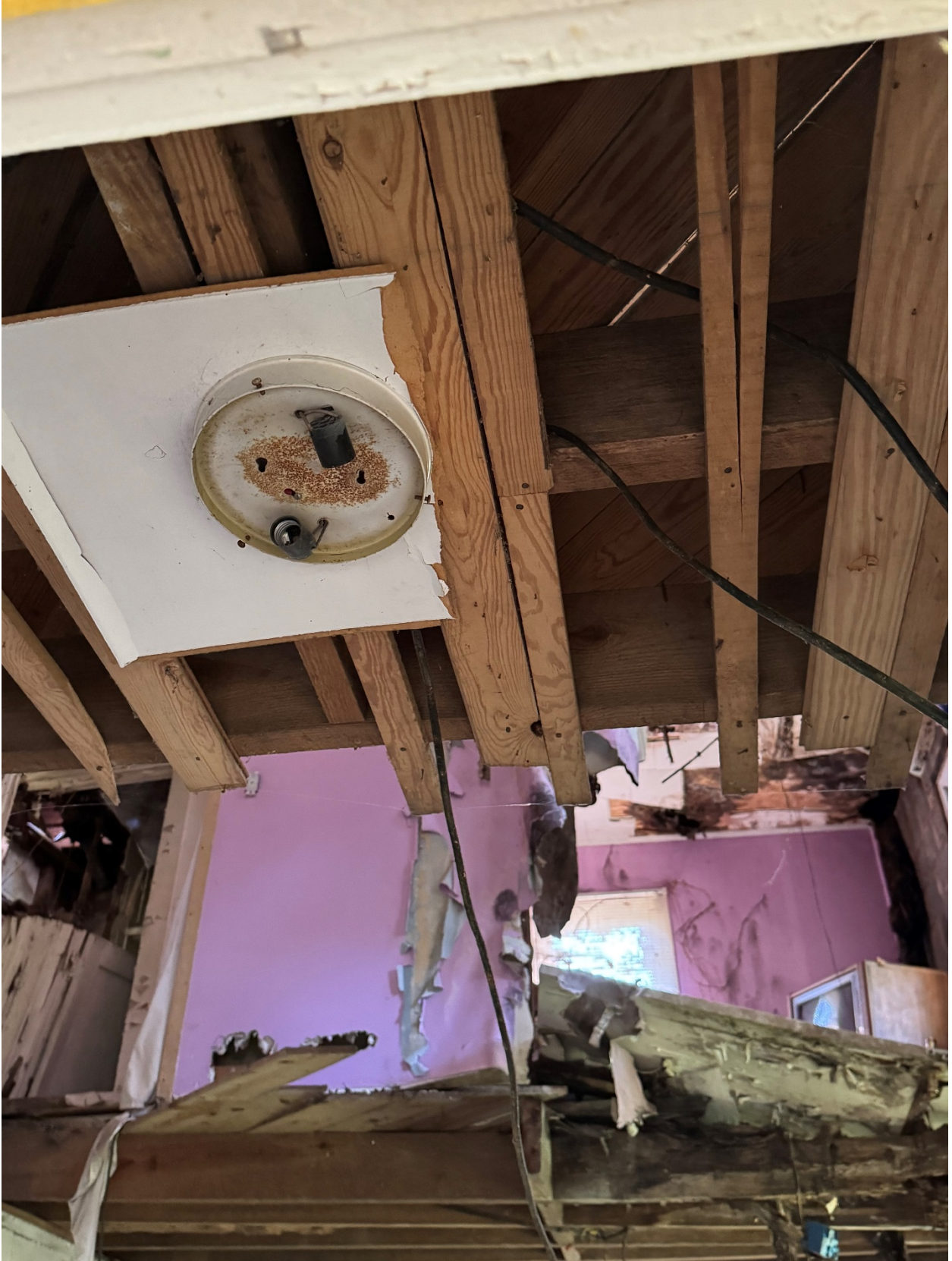
Photo from 2025 Floor collapse
