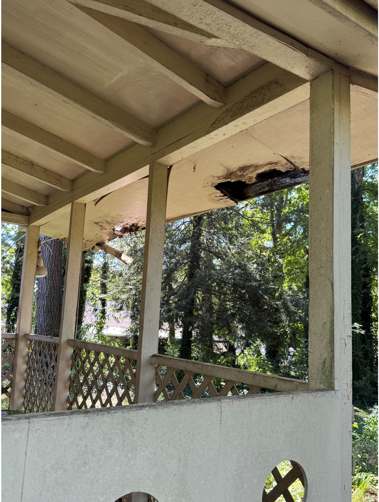
Rear Porch Rot
