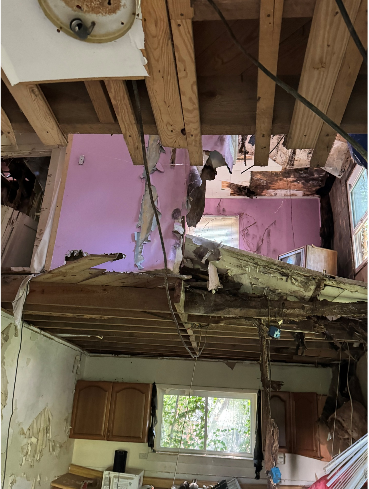
Photo from 2025 Floor Collapse
