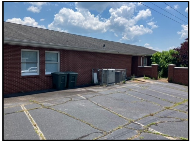
Above: Back of Beall Hall where exterior doors will be required for egress
