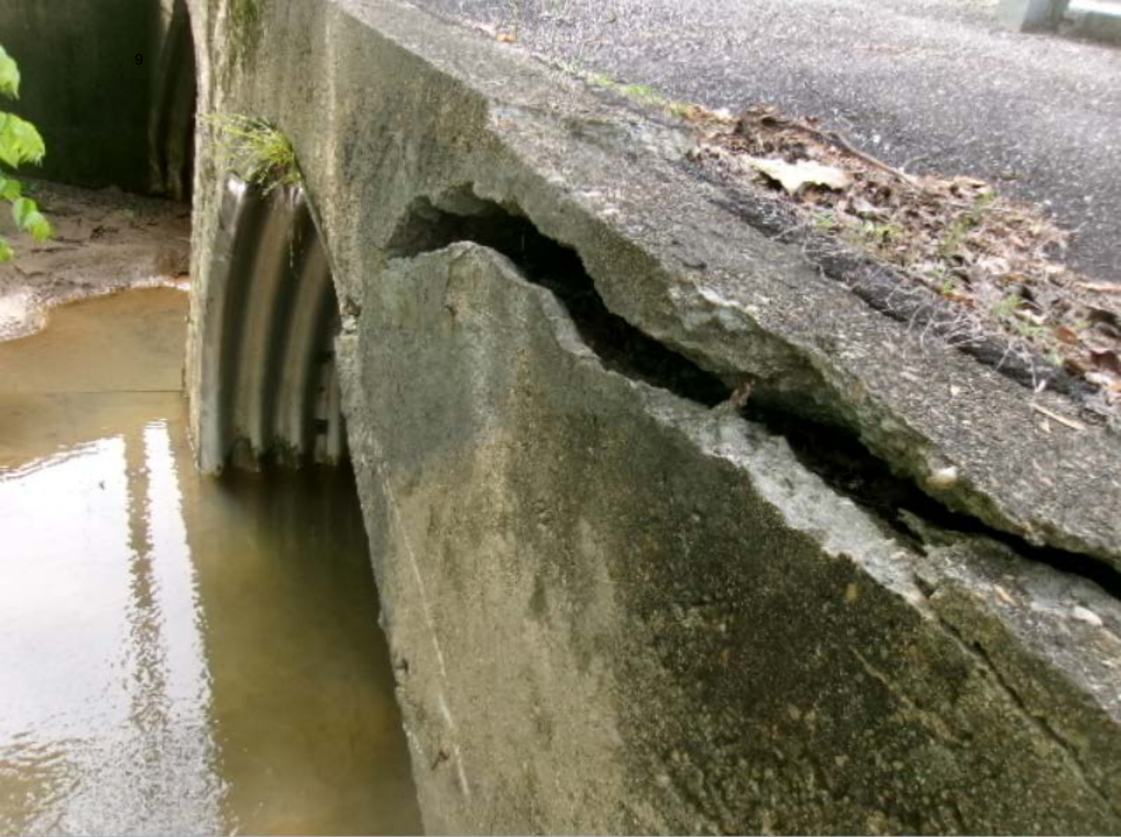
PAR: 5 FEET LONG X 2 FEET TALL X FULL WIDTH SPALL WITH EXPOSED REBAR AND SHIFTING IN EAST HEADWALL OVER BARREL 2
