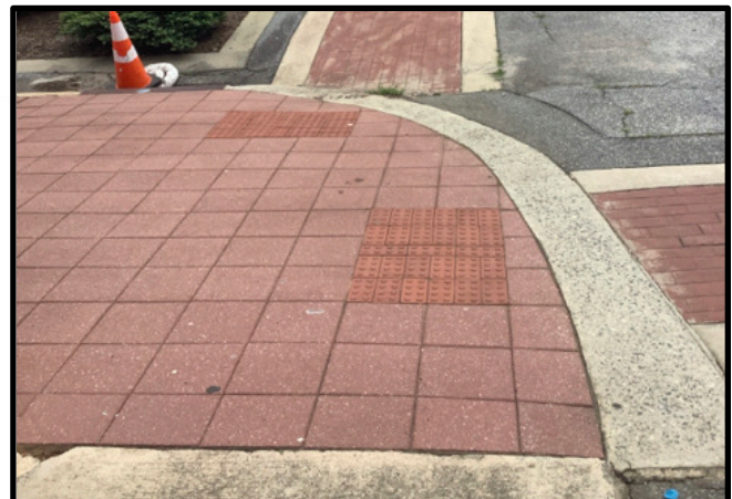
Deficient Curb Ramp (Slope)
