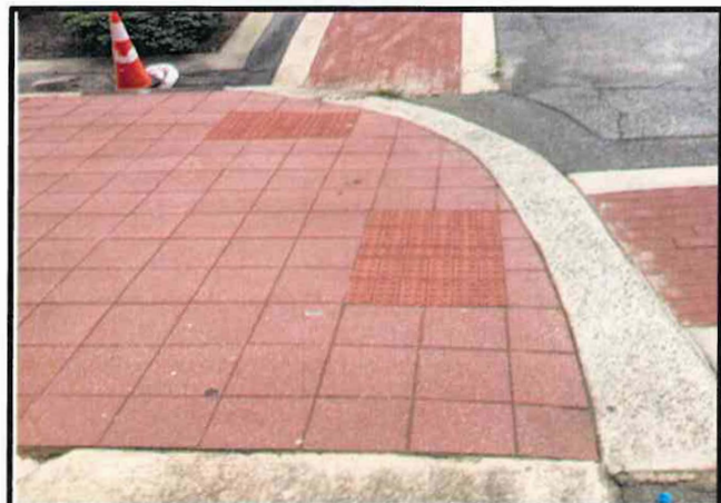
Deficient Curb Ramp (Slope)
