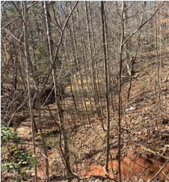
Erosion and channelization (foreground) on Lot 13; sediment basin holding water following 1" storm event (background).
