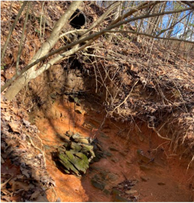
Erosion on Lot 29 below the outfall
