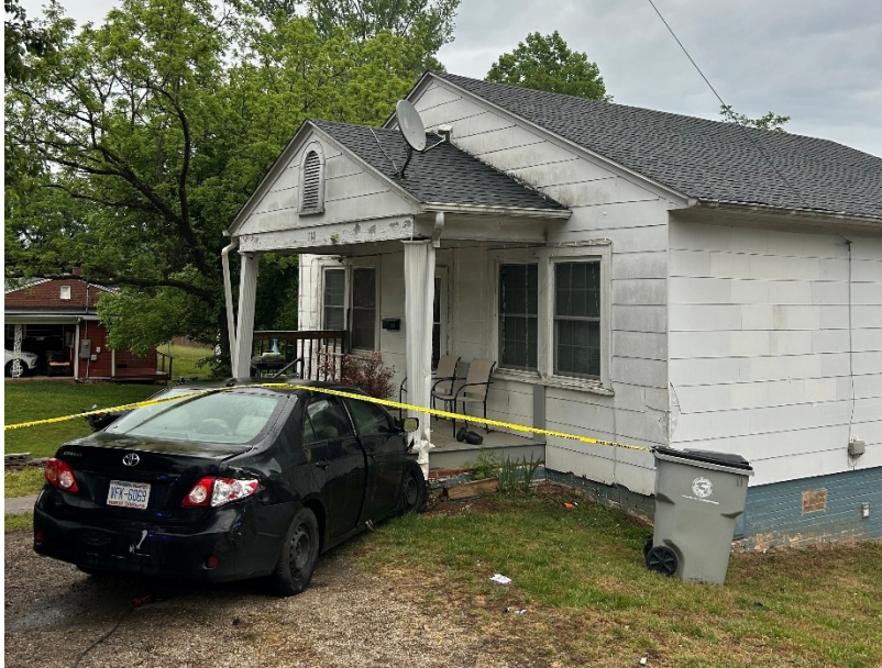
Pennton Ave. car hit house.
