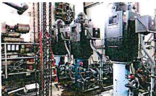
Cahah's Pump Station
