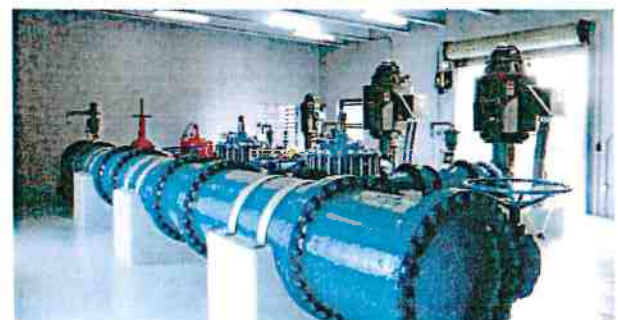
Whitnel Pump Station
