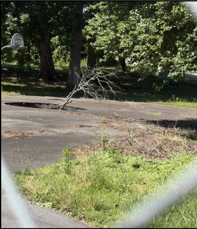
Above: Sinkhole on basketball court adjacent to playground
